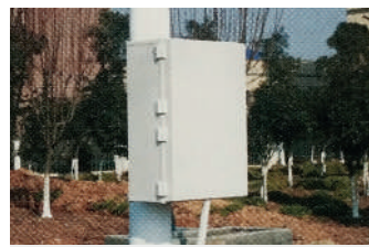
Fixed on the telegraph pole
